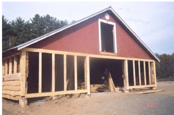
The barn has been renovated to serve as an equipment storage facility. Photo by Sarah Clarkin
