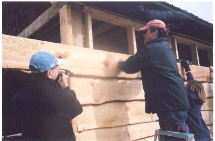
Volunteers Fred Cady, Pieter Litchfield and Jill Litchfield side the new equipment storage facility at 80 Scout Road. Photo by Sarah Clarkin
